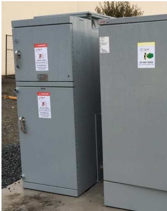
Picture 9 – Customer-Owned Dead Front Kiosk with Both Doors Closed
