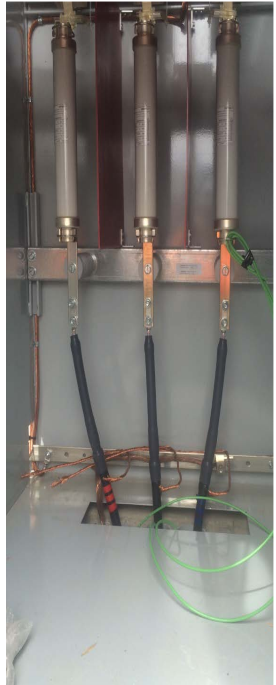
Picture 6 – Customer Fuse Compartment with Customer Primary Service Cable Terminations
