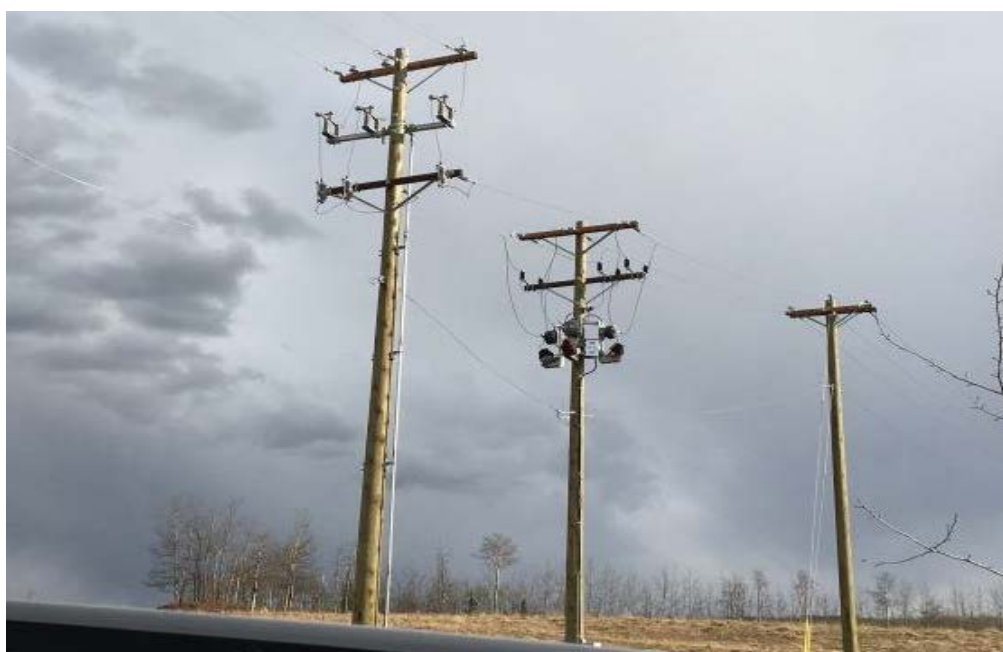
Picture 8 – Customer Service Switch and O/C Protection on First Pole and BC Hydro Primary Revenue Metering on Second Pole
