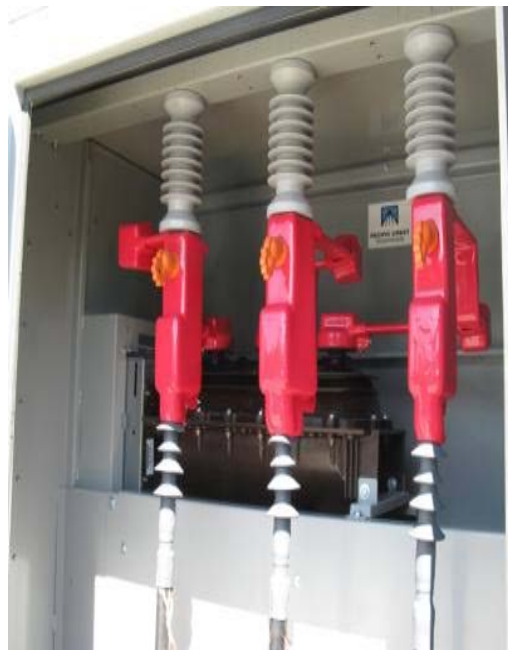
Picture 2 – Utility Service Cable Compartment Showing Disconnect Switch and Primary Bus Work
