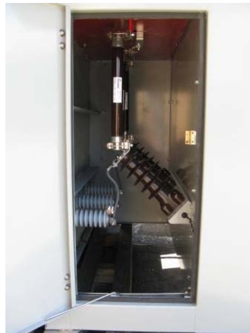
Picture 4 - Customer-Owned Primary Service Fuse Compartment
