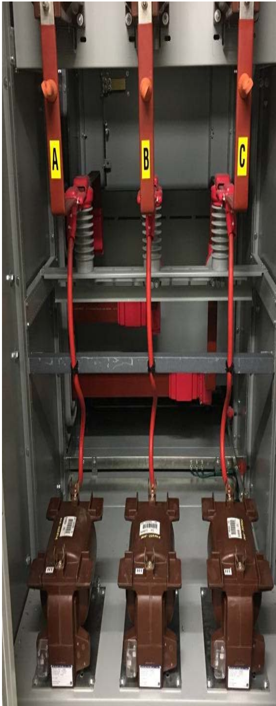
Picture 5 – Primary Revenue Metering Compartment
