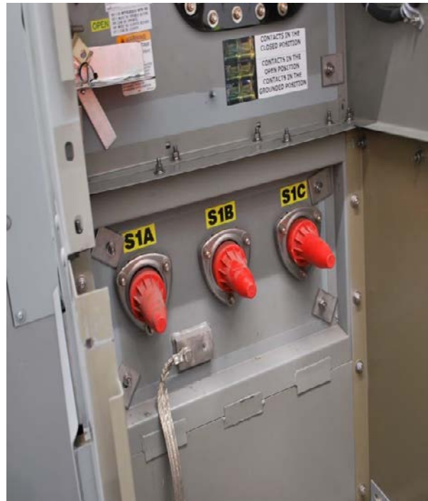
Picture 10 - Dead Front Kiosk with Both Doors Open - Showing Grounding Switch Above and Service Cable Bushings Below
