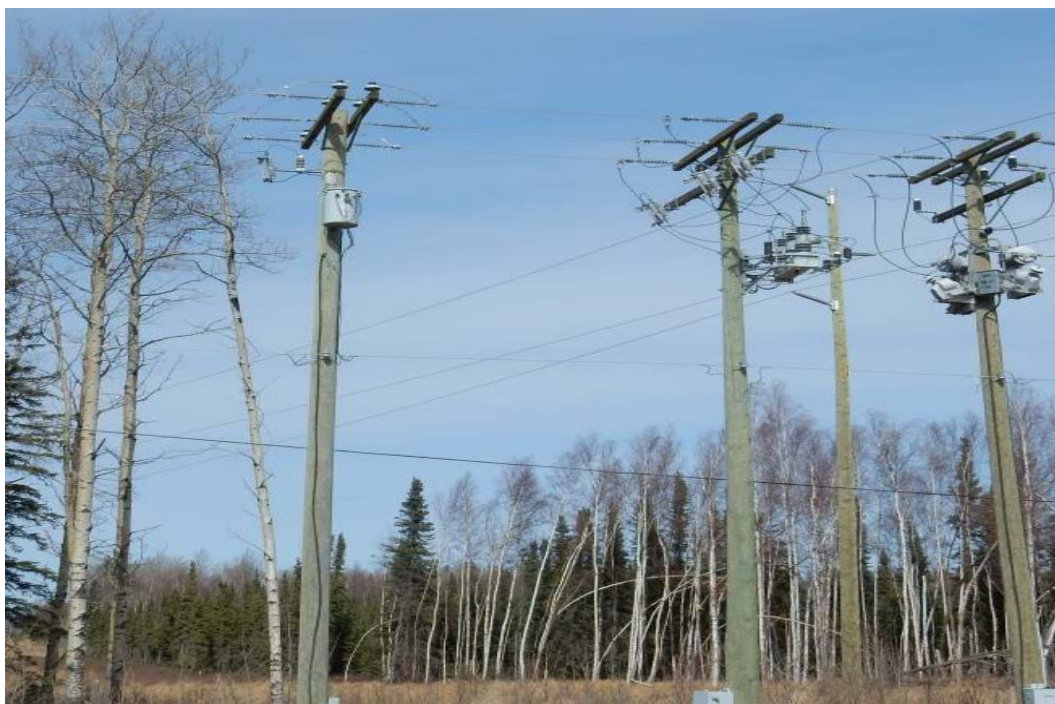
Picture 7 - Customer-Owned Recloser and BC Hydro Primary Revenue Metering
