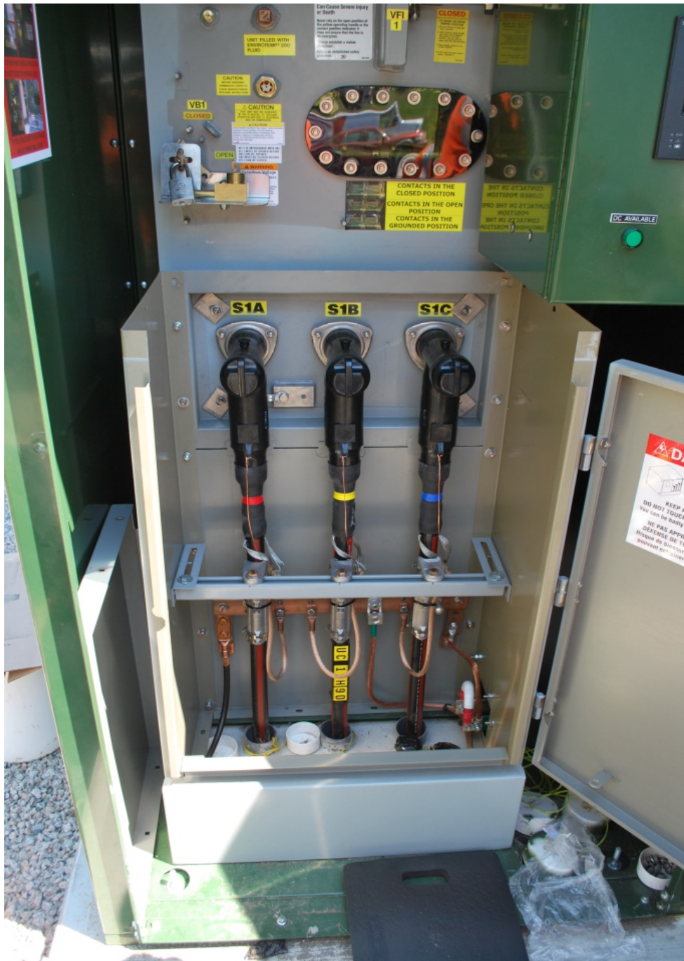
Picture 12 – Close-Up of Dead Front BC Hydro Utility Service Cable Compartment with Terminators, Cable Supports and Grounding
