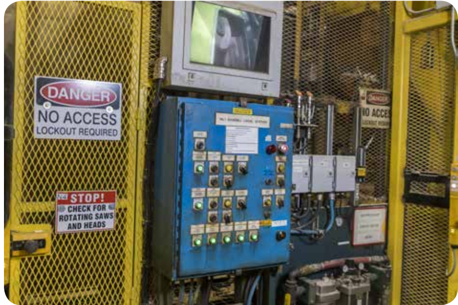
Figure 9: Control power panel.
