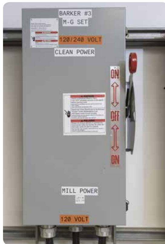
Figure 10: Electrical boxes or panels should be labelled or marked to indicate the machine, equipment, or process supplied and the energy type and magnitude.
