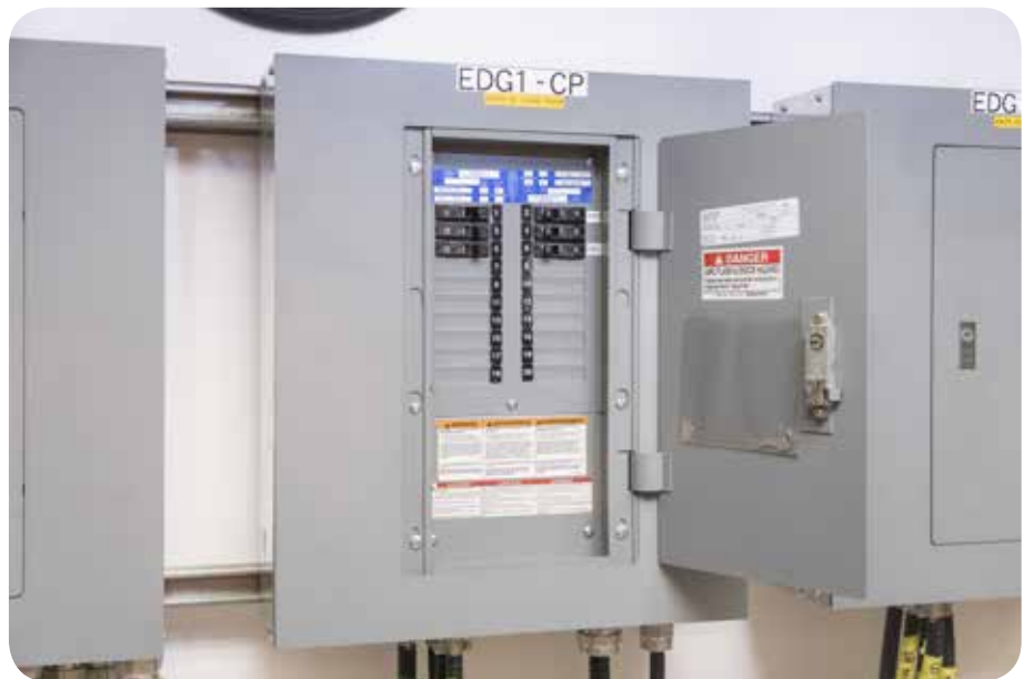
Figure 8: Main power panels — circuit breaker panel.
