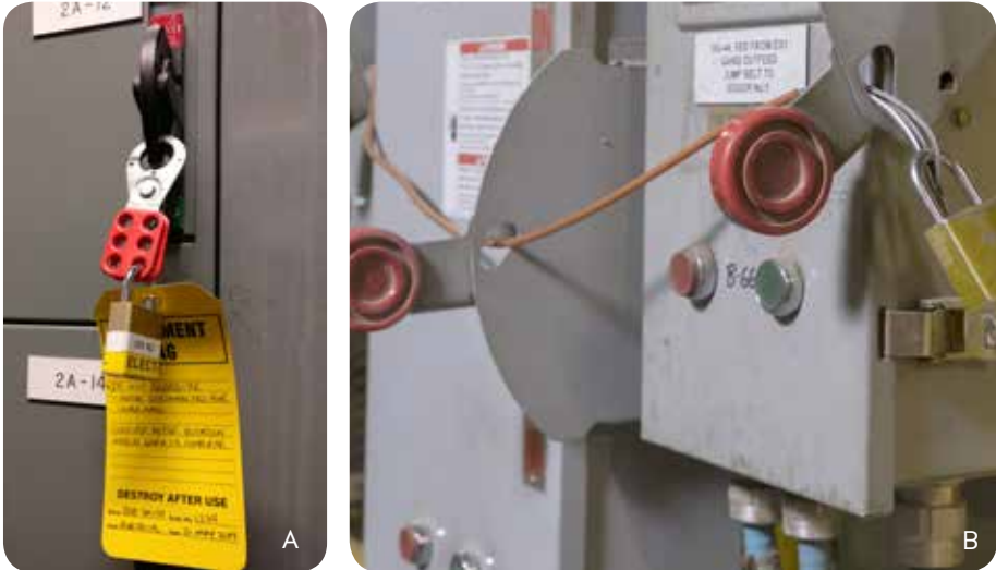
Figure 14: (A) A lock with a tag. (B) A cable lockout.
