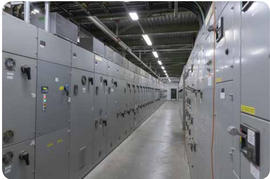
Figure 7: Main power panels — motor control centre.
