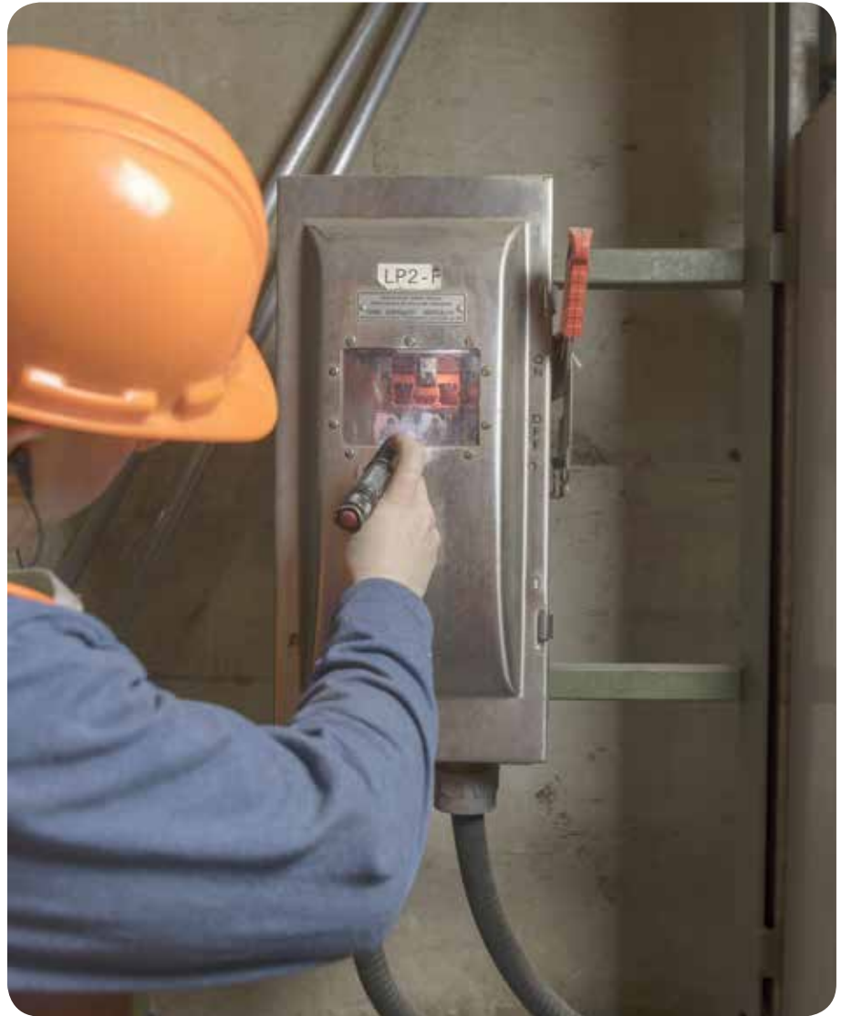
Figure 5: A worker observing the blades disengaging in a visible blade disconnect switch (visi-disconnect) panel.
