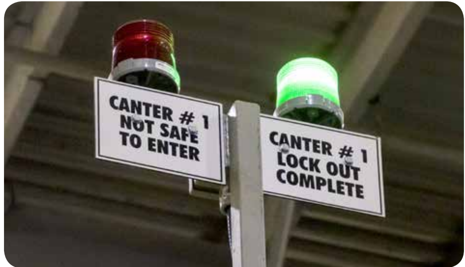
Figure 6: An indicator showing that it is safe to enter the area.
