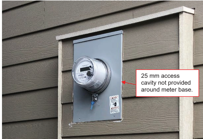
Figure 8. Non-compliant installation with no access cavity around meter base
