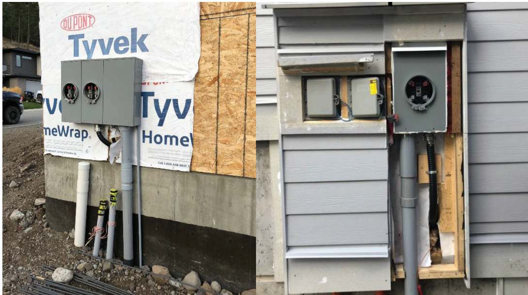
Figure 4. Option 1 – Outside of building wall, ready for inspection and connection, covering to be installed after connection
